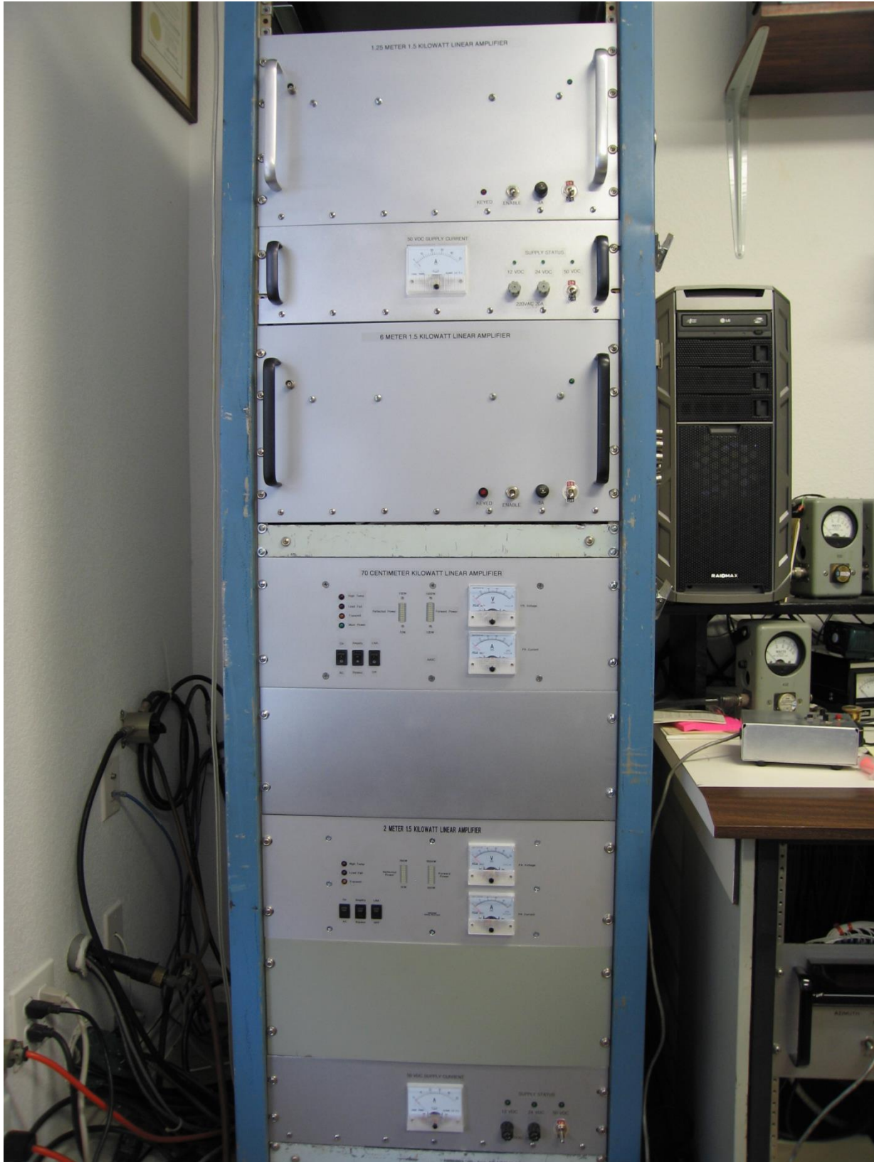
Figure 5 AA5C LDMOS KW Amplifier Rack
