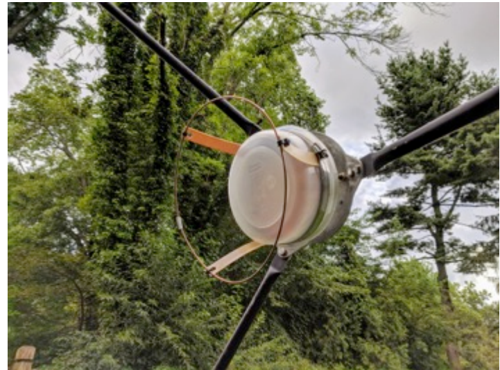
Installed in TVRO Dish
