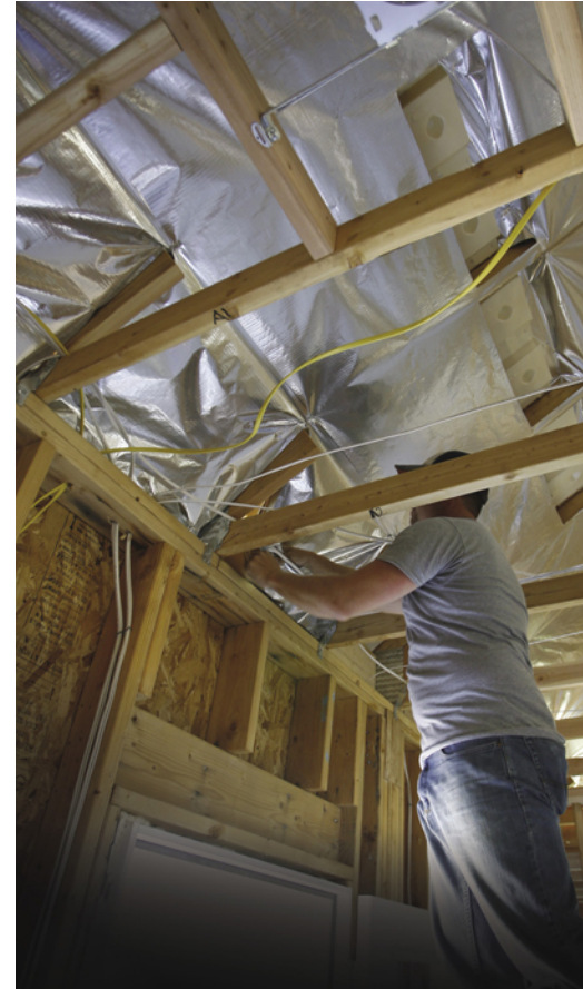
Radiant Attic Insulation
